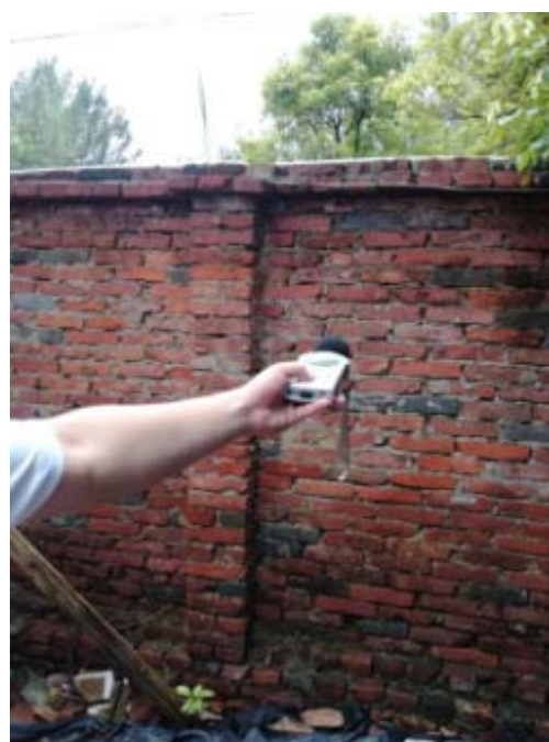
1#厂界南侧外1米处
